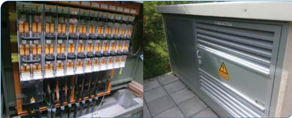
Fig. 2 Example of low-voltage substations used in Hittistetten (Attribution: SWU Netze)
